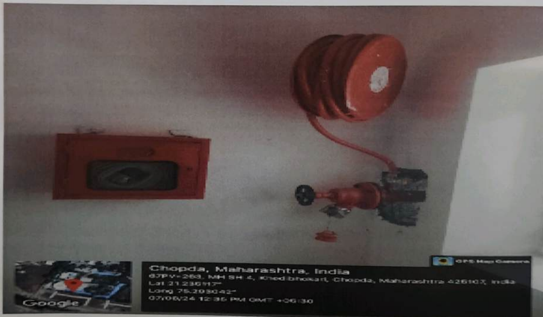
Fire Fighting System
